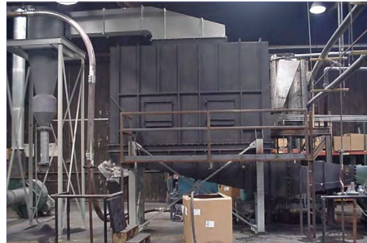
Continuous Fluid Bed Dryer
