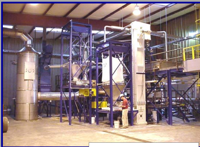
Large -Scale Pilot Plant
