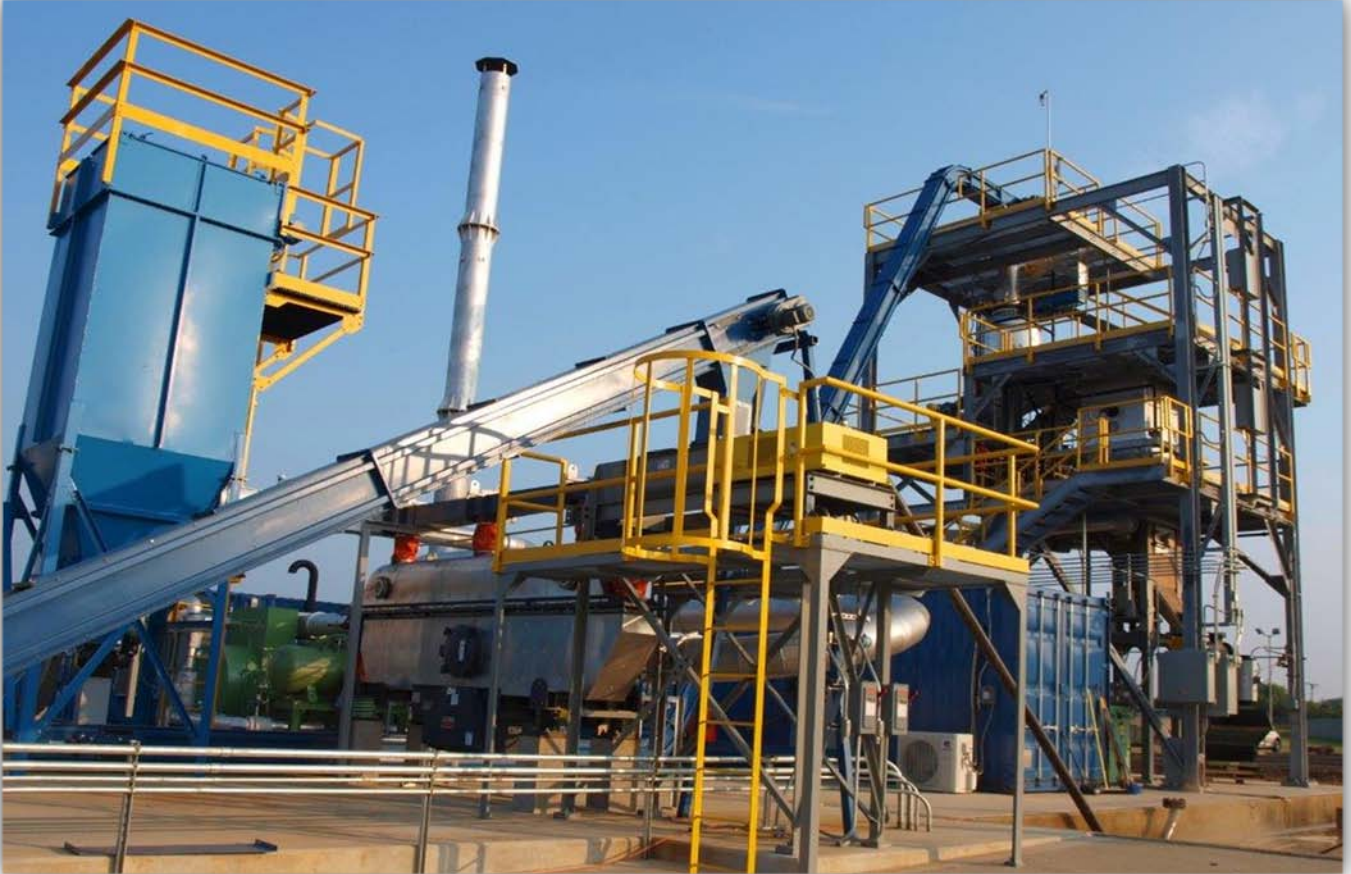
Photo: PHG Energy - Covington, TN Gasification Facility - 2014
